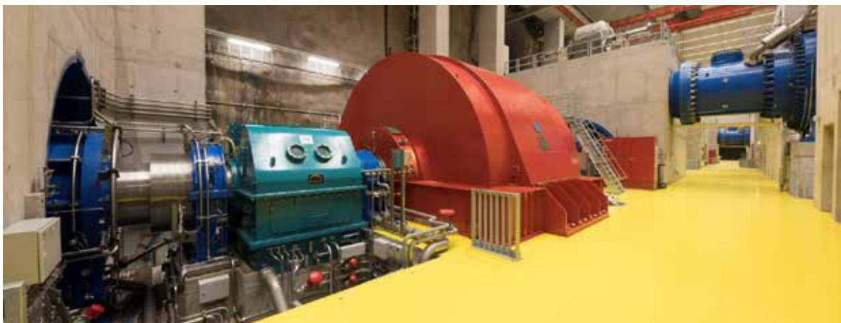
With the expansion of renewable energy sources, electromobility and smart grid technologies, illwerke vkw is making a contribution to Vorarlberg's energy autonomy. The photo shows the Obervermuntwerk II on the Bielerhöhe, which opened in 2019. ©Patrick Saely/illwerke vkw | TOP Sustainable mobility is one of Vorarlberg's environmental objectives. ©Manuela de Pretis/WISTO
